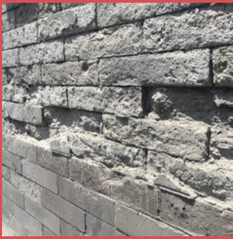
Old bricks damages
