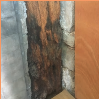
Wood rotting (columns footing)
