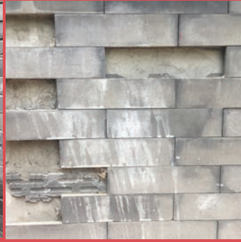
Falling brick veneers
