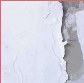
Interior lower walls humidity
