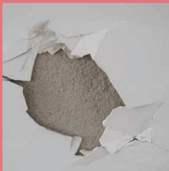
Falling plaster and paint peeling
