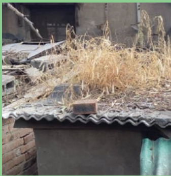
Low quality construction
